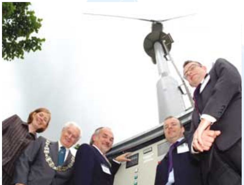
Left to right are Rose Gardner, Npower, Clifford Wilson, North Yorkshire County Council, Alan Harrison, Yorkshire Water switching on the wind turbine, Stuart Mason, Head teacher, Nidderdale and Chris Roberts, Clear Skies.
